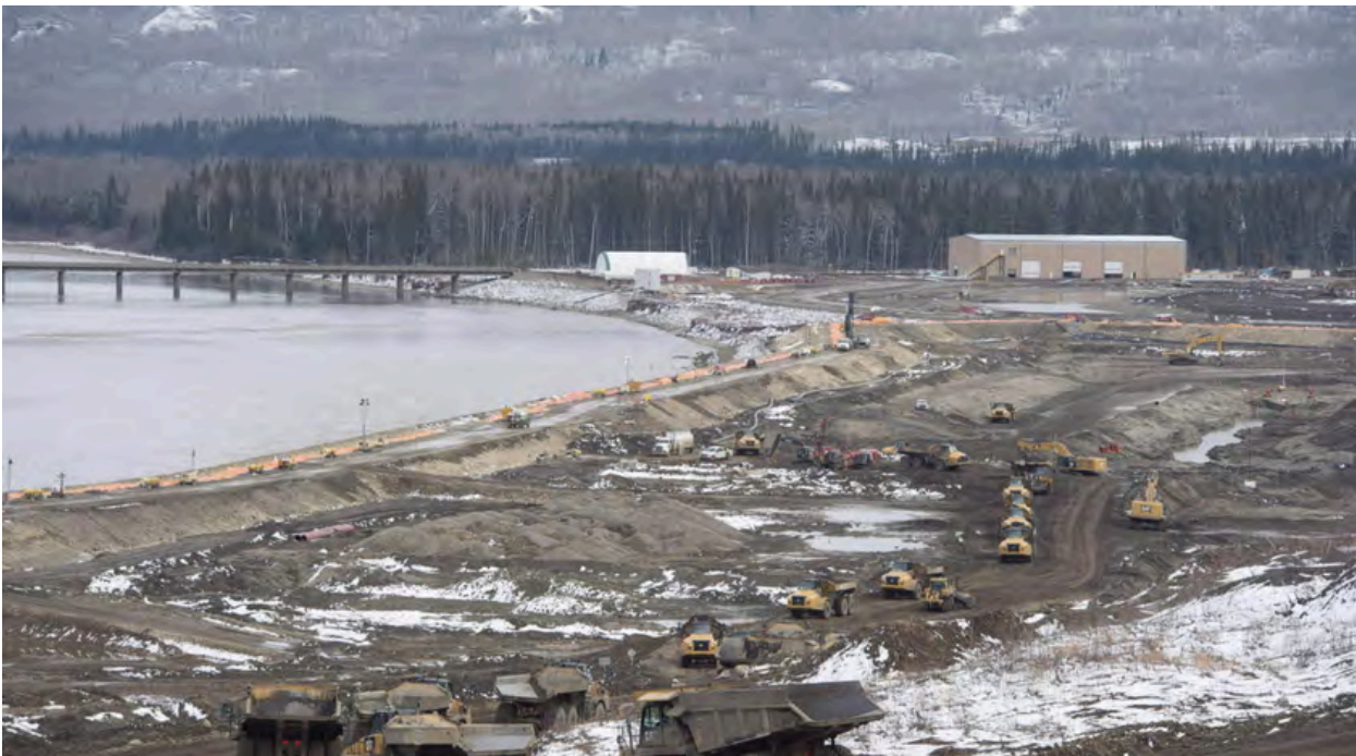
The Site C dam location is seen along the Peace River in Fort St. John, B.C., in April 2017. (The Canadian Press/Jonathan Hayward; as cited in Desmarais, 2018)
